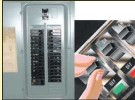
The photo above shows a typical circuit breaker panel with switches that indicate if the circuit is on or off.
