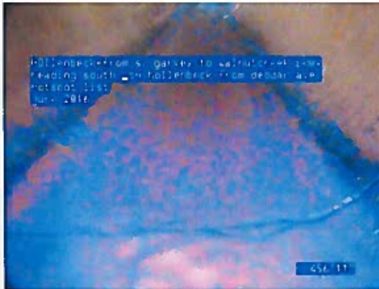
Figure 4—Crack in Channel Mainline on Hollenbeck Ave
