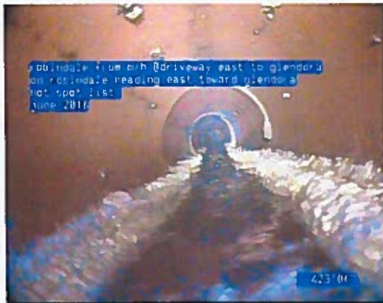
Figure 1 – FOG Buildup in Mainline on Robindale St
