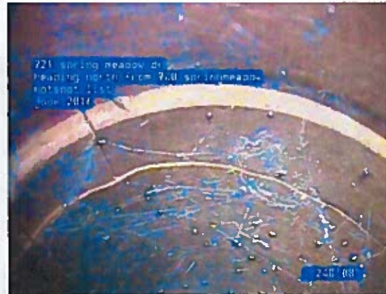
Figure 5—Crack at Joint Mainline on Spring Meadow Drive
