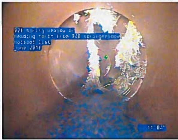
Figure 6—Root Intrusion Mainline on Spring Meadow Dr
