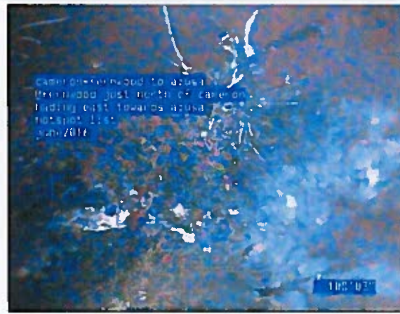
Figure 7—Roots and FOG Lateral on Cameron Dr
