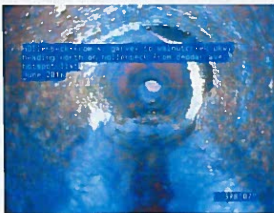
Figure 3—FOG Buildup in Mainline on Hollenbeck Ave
