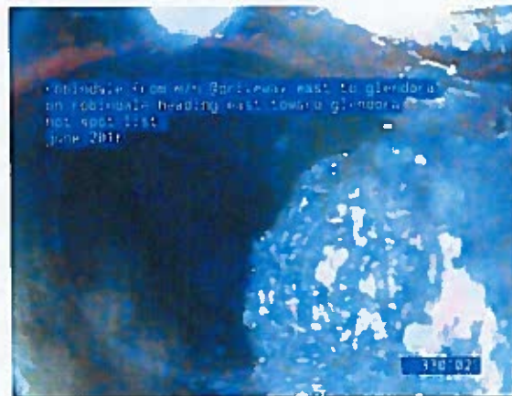
Figure 2 –FOG Buildup in Lateral on Robindale St
