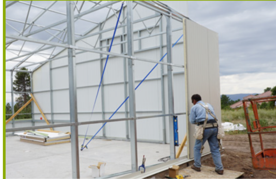
Installation of a south sloped PV Greenhouse with insulated North and West walls with radiant flooring for year round crop production
