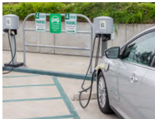
Electric vehicles charging stations at the Civic Center
