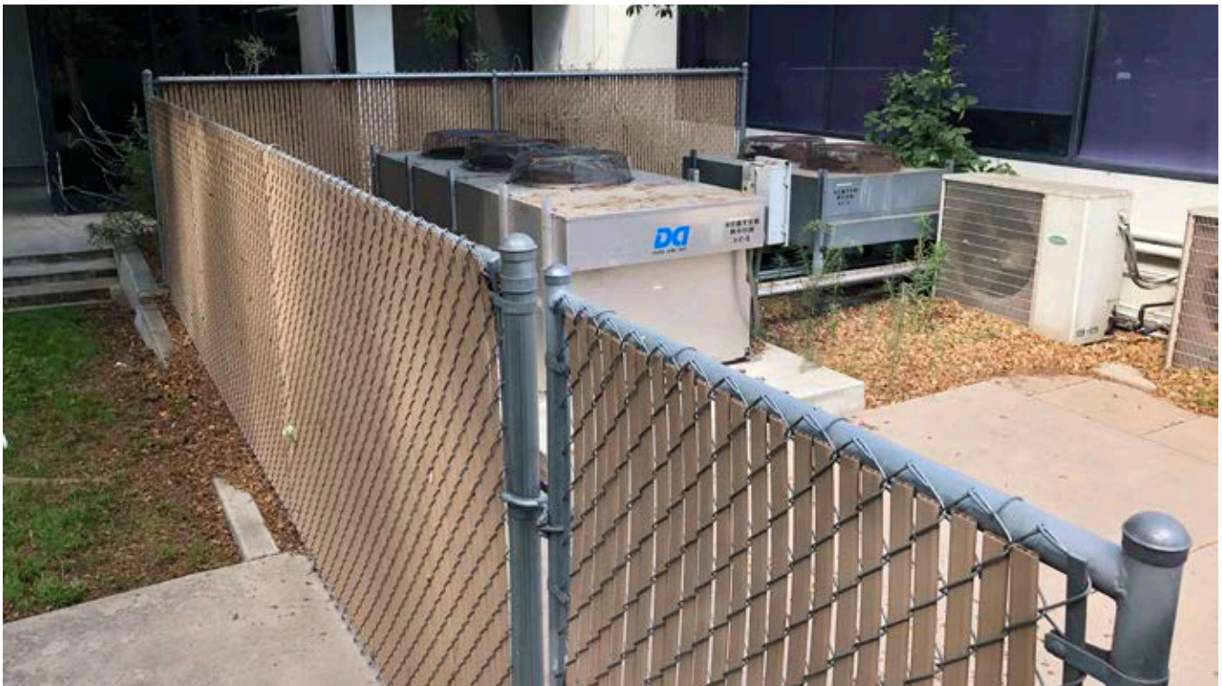
Ground-Mounted Mechanical Equipment Screened Behind a Fence
