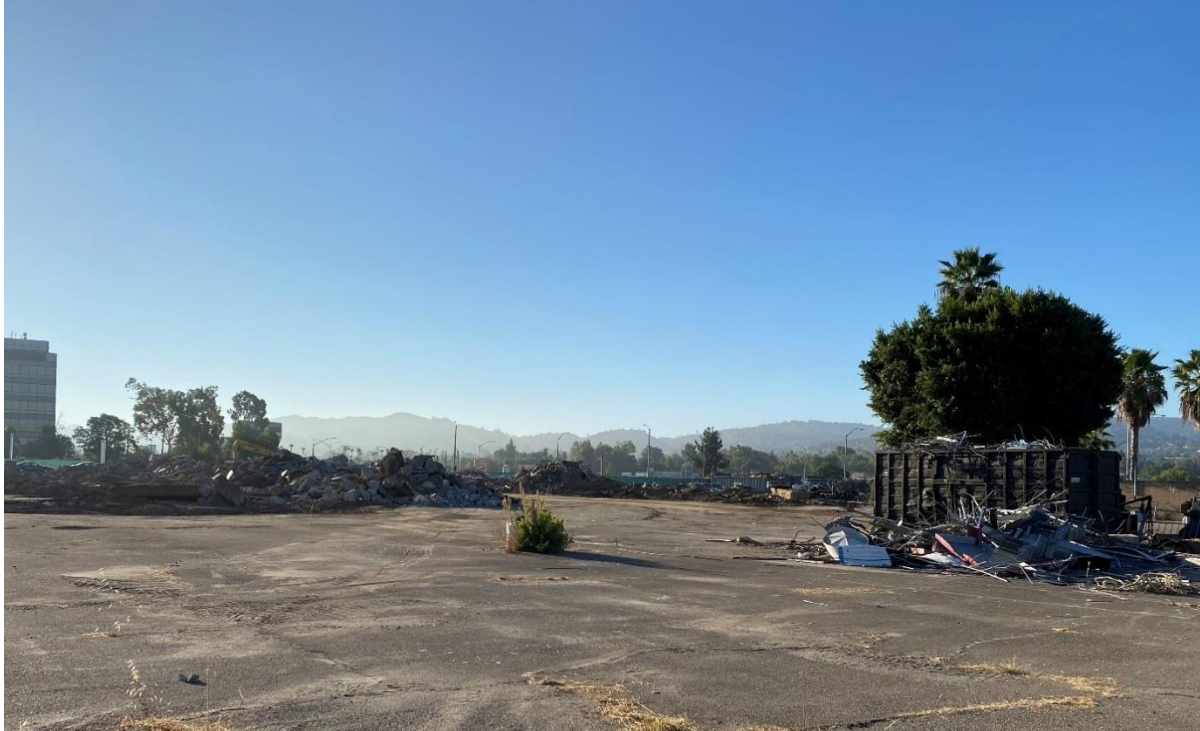
View of project site and demolished materials pertaining to former auto dealerships.
