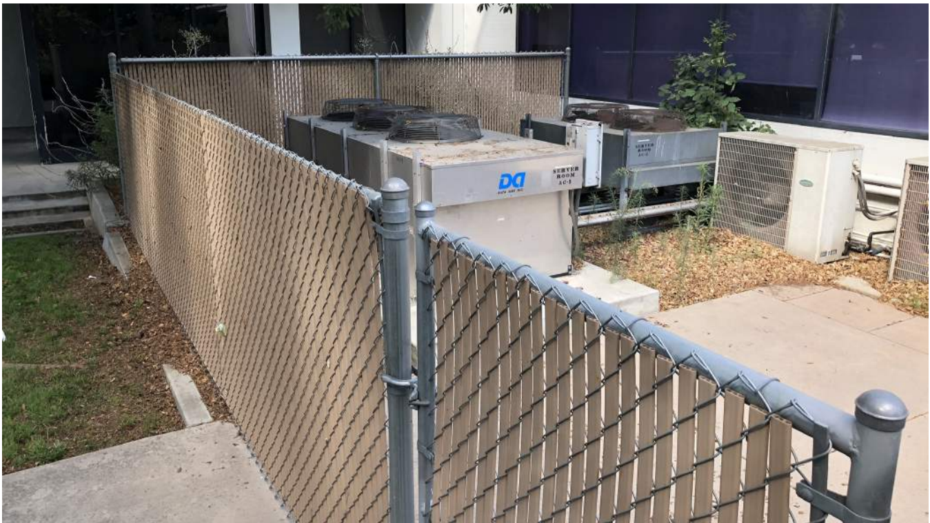
Ground-Mounted Mechanical Equipment Screened Behind a Fence
