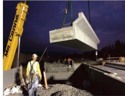
Overhead protection is required when moving heavy objects over Metro ROW or in areas designated for public use.
