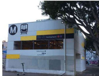
Constructed above is a wooden box over the entrance portal for overhead protection at the 4th/Hill Station.
