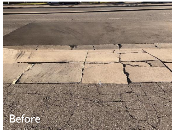
919 N. Sunset Avenue | Broken Driveway Approach Repair
