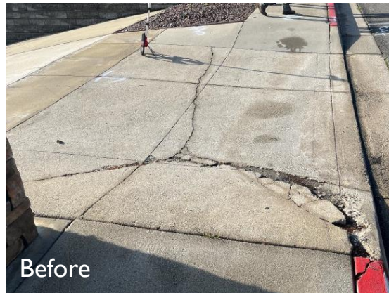
404 S. Citrus Street | Broken Driveway Approach Repair
