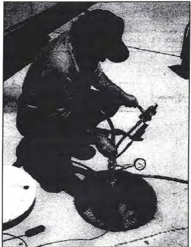
FIGURE 4-4. The plumber’s plug provides a leak-tight connection to draw a vacuum on the tank interstitial space.
